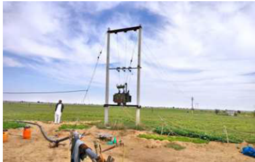
Possible pathways to address poor quality of electricity supplied to agricultural consumers were also discussed. SPECIAL ARRANGEMENT
